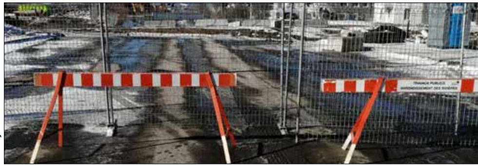
This barrier greets motorists on Boul. Pierre Bertrand at Rue Beaucage. Workers are replacing damaged water pipes.
